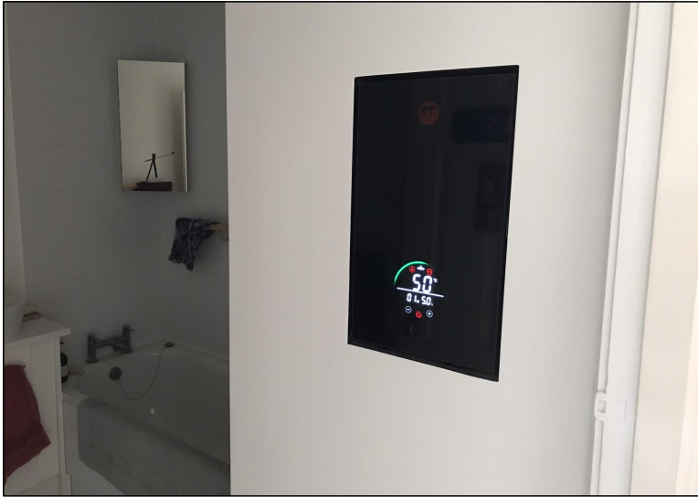
And this is the new eclectic boiler, sunk into the wall, looking very high-tech!
